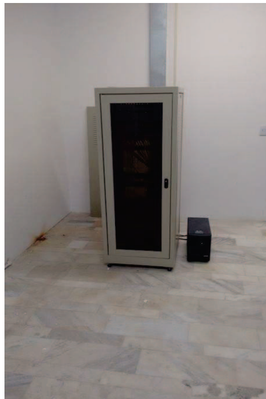
Rack do subsolo
